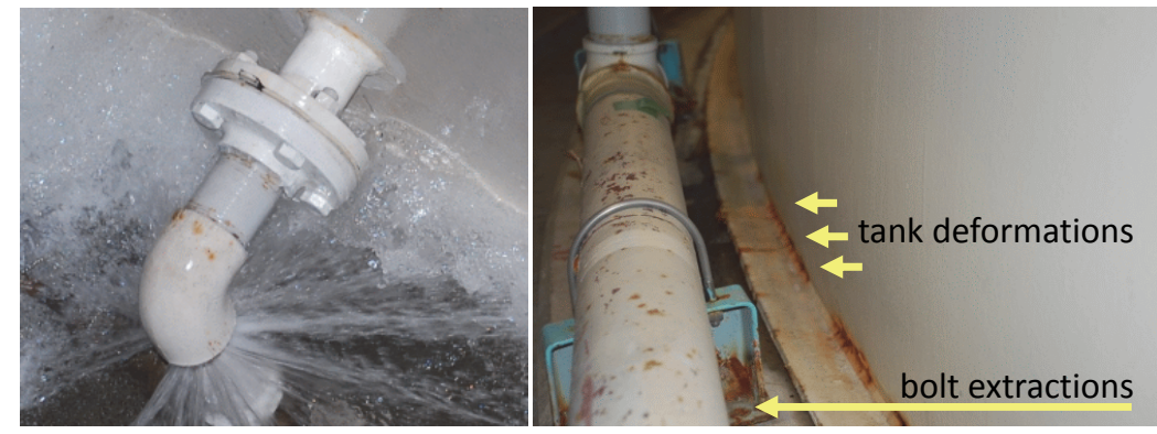
Fig. 7 Tank deformation and pipe bolt extractions. Earthquake damage. It took 3 days for the water to drain.
